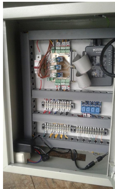
Figure 6. Control Panel for Prototype of the Mechanical Seal Test System using NI MyRio
