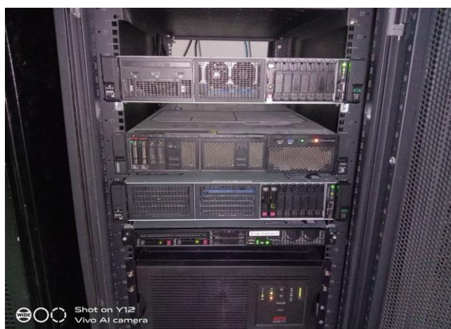
Fig. 3 Server Deployment Location
