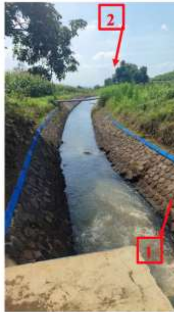
Fig. 1 Deployment of IoT Device Node 1 and Node 2
